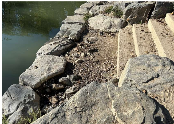
Behind-the-boulder edging erosion at third access point
