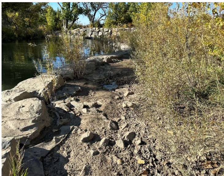
Behind the boulder edging erosion
