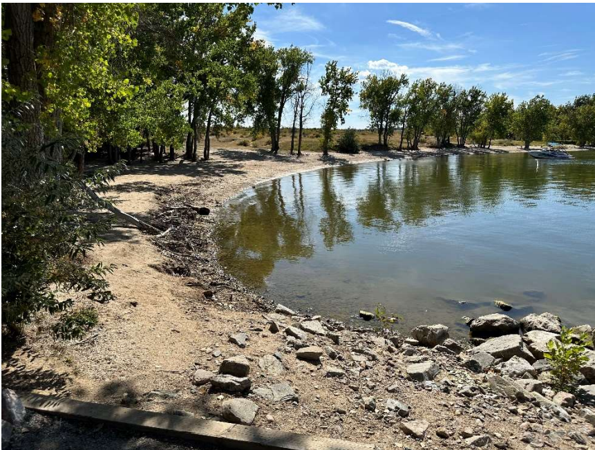
100-foot eroding shoreline that will be stabilized by current maintenance project.
